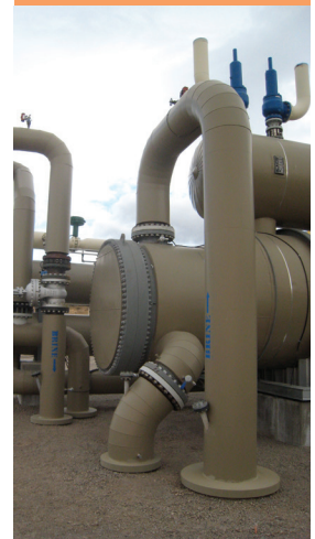
Geothermal piping, Steamboat Springs, NV
