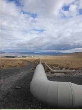
Geothermal piping, Fallon, NV
