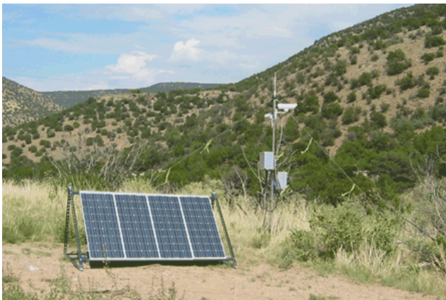
Fig. 5. Assessment Equipment Solar Array Power Supply
