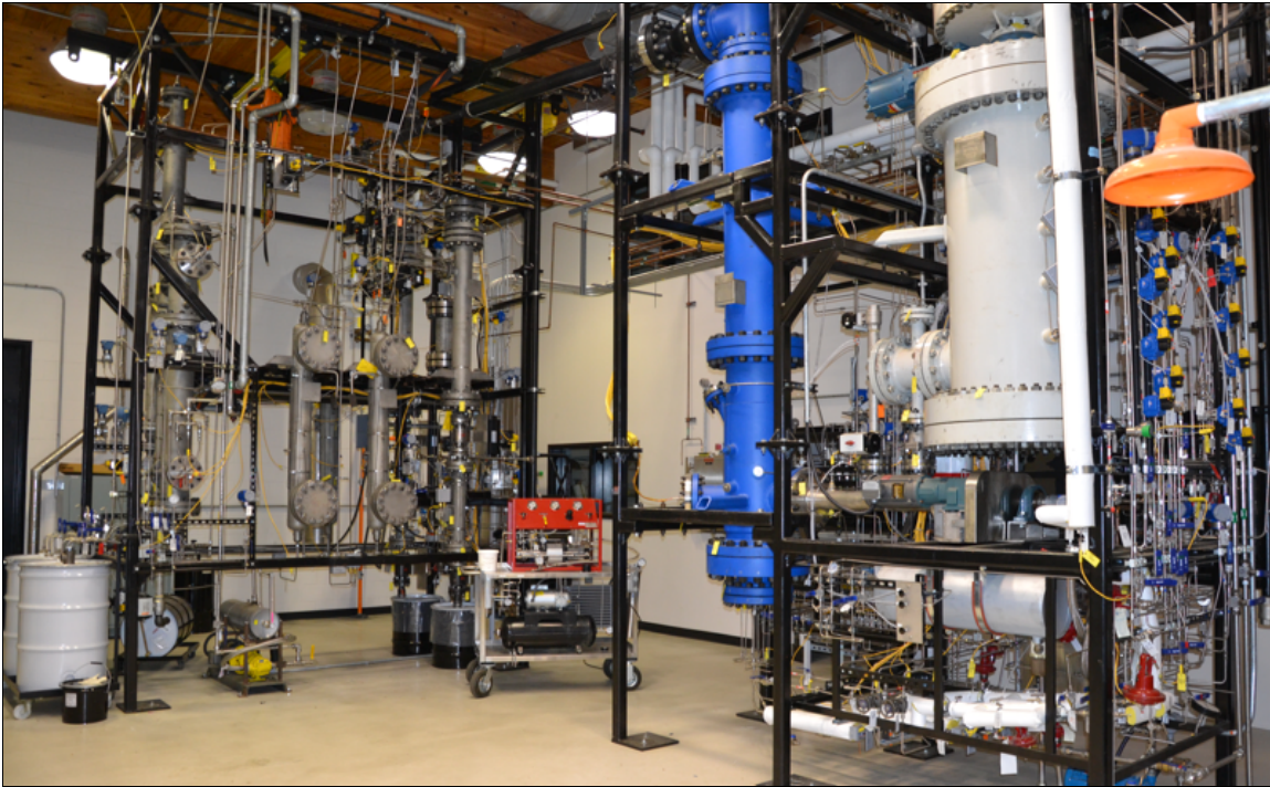
Overall view of gasification platform (right) and gas conditioning platform (left).
