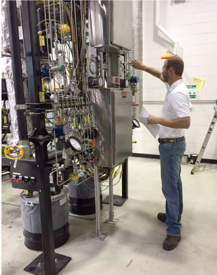
Performing pre-run check of gas conditioning system.
