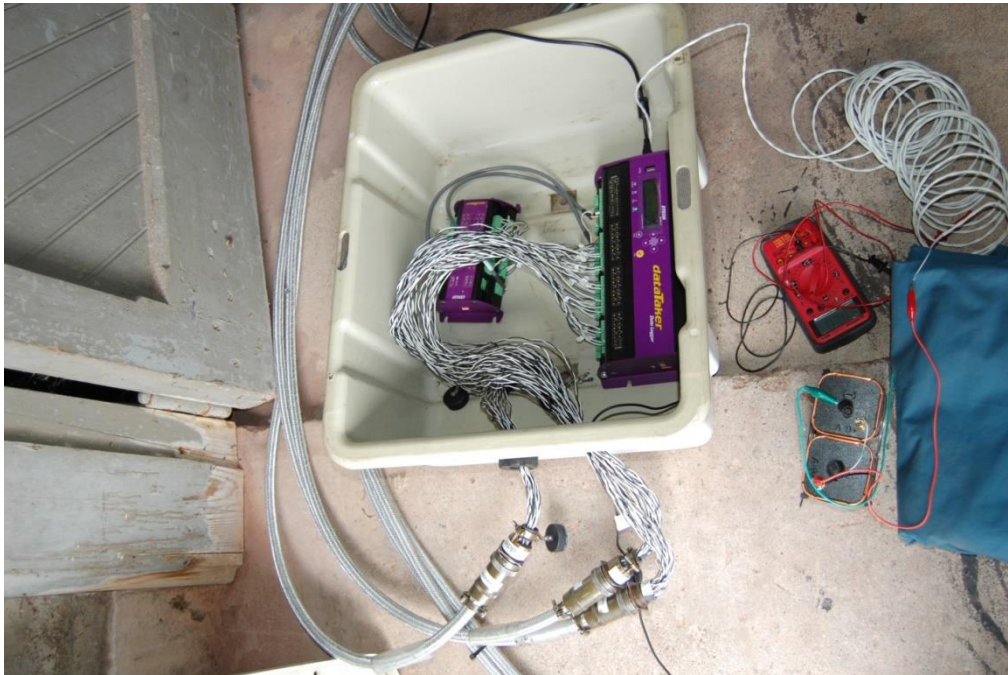
Figure 9.6 IFMS DT85M data logger with built-in cellular modem and CEM20 extension module; shown during installation and test, resting on the South Light's floor.
