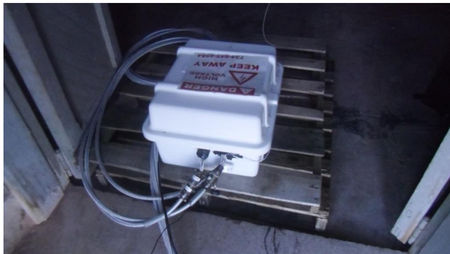
Figure 5.4 IFMS Data Logger housed within the lighthouse superstructure.
