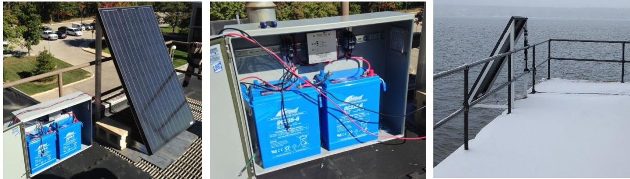
Figure 9.3 [Left] Solar panel and battery box [Middle] Batteries and solar power condition circuitry in battery box [Right] Solar panel mounted on the south side of the lighthouse.
