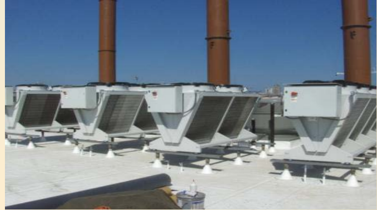
Engine radiators in place over Engine Room.
