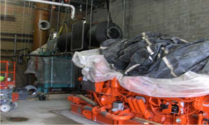
Showing engines, heat recovery units and silencers.
