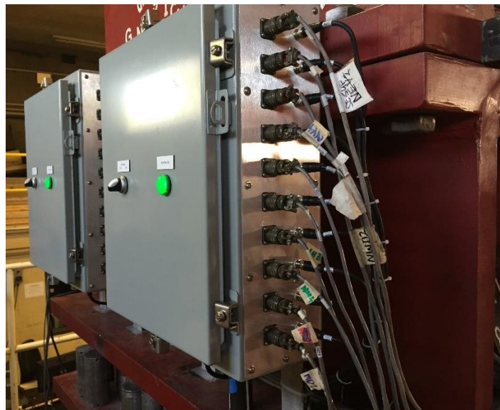
Figure 177. New power supply boxes for LVDTs
