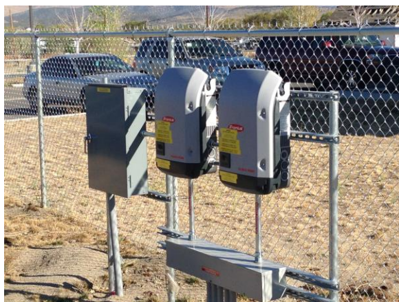
Installed inverter and electrical components
