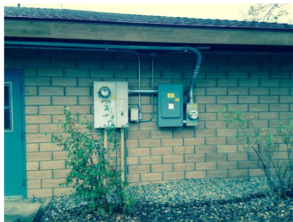
Installed solar meter and junction box
