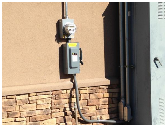
Installed solar meter and junction box
