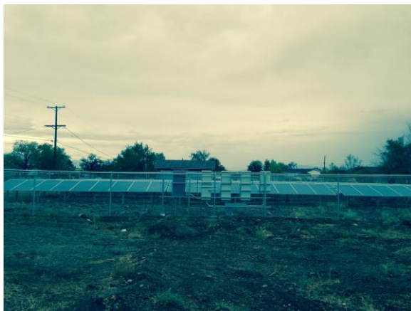
Completed solar array and fencing
