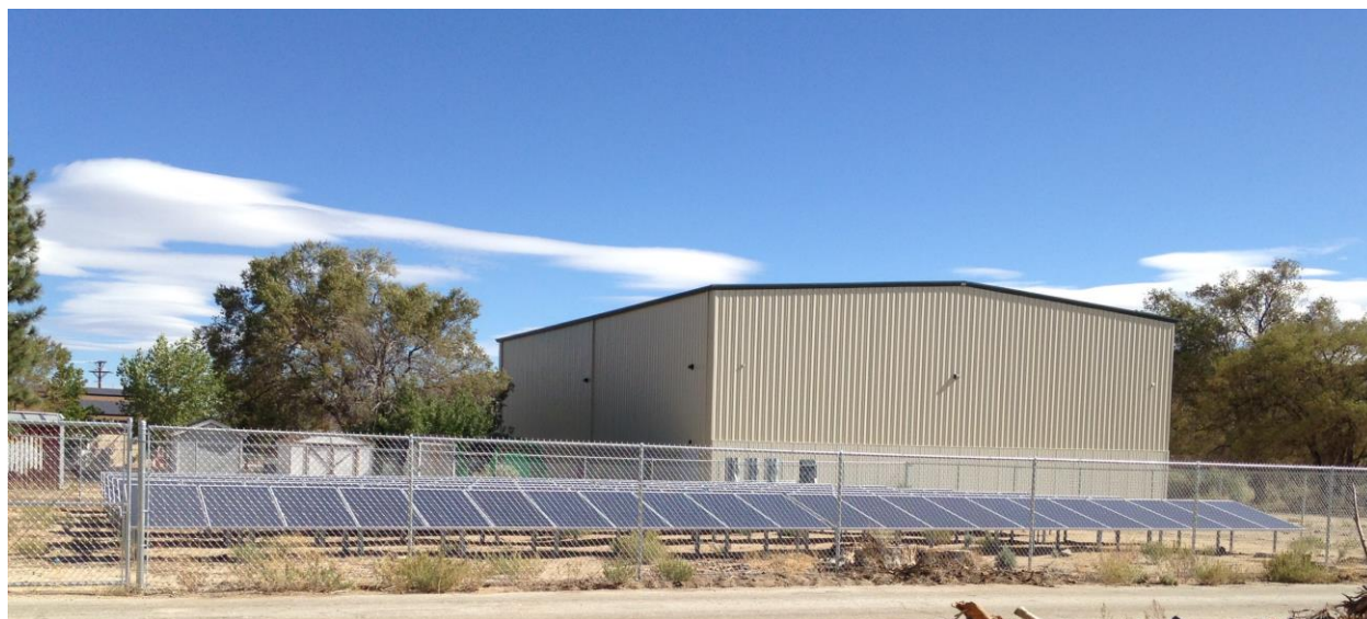
Completed solar array and fencing
