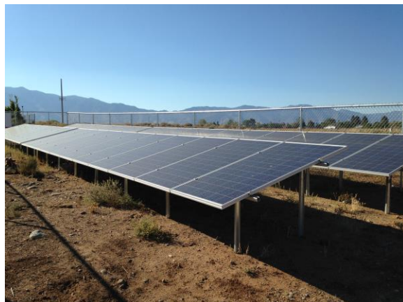
Completed solar array and fencing
