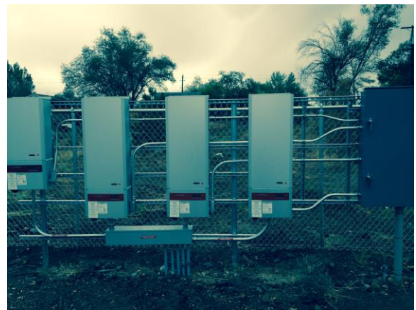
Installed inverter and electrical components
