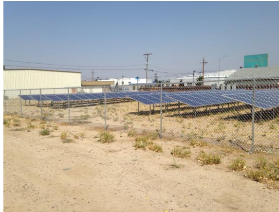
Completed solar array and fencing
