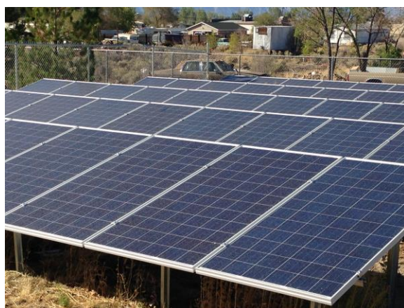
Completed solar array and fencing
