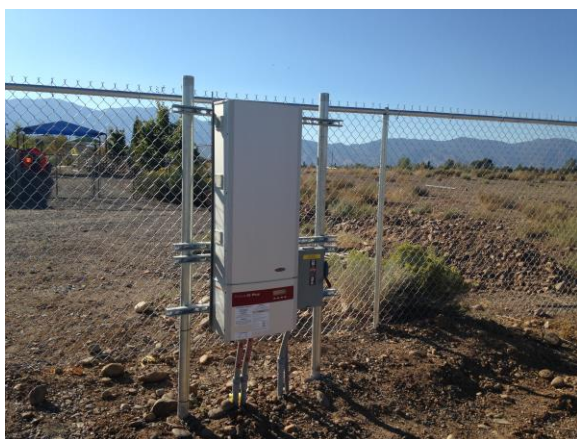
Installed inverter and electrical components
