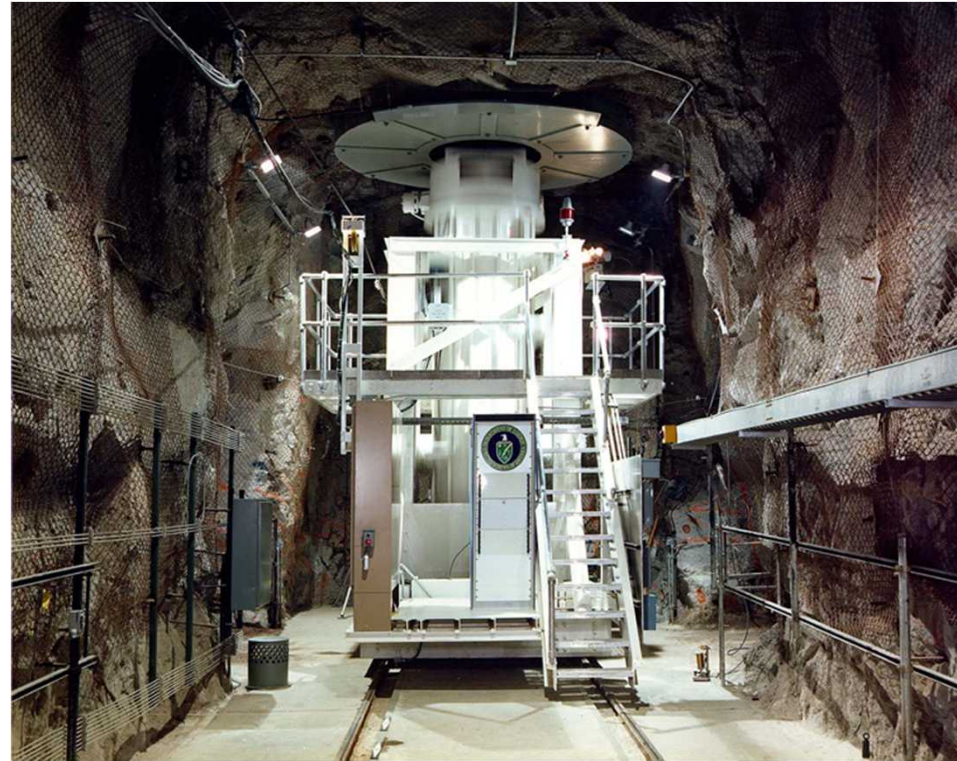
Rail-mounted canister transfer and emplacement machine, main gallery (in receive position under waste handling borehole)
