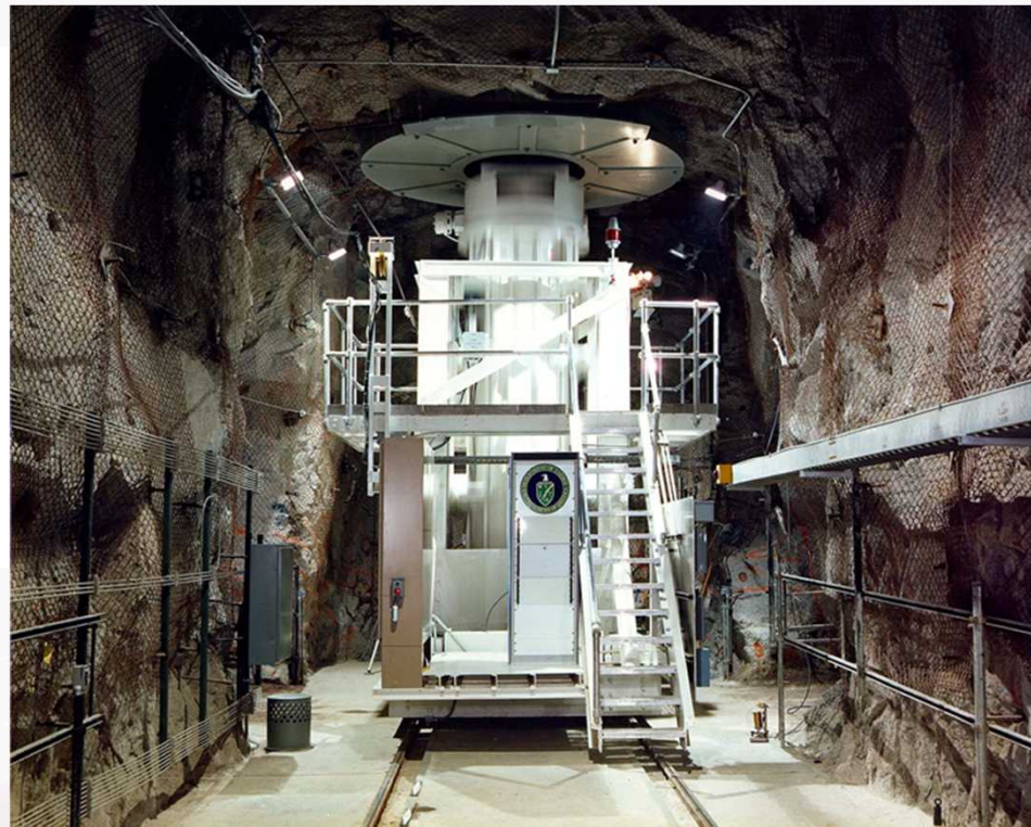
Rail-mounted canister transfer and emplacement machine, main gallery (in receive position under waste handling borehole)
