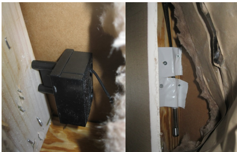
Figure 22. Moisture content and temperature/relative humidity sensors mounted in wall cavity
