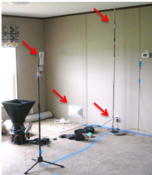
Figure 34. High, low, and primary room temperature sensors
