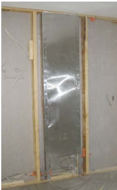
Figure 33. Vertical transfer fan duct
