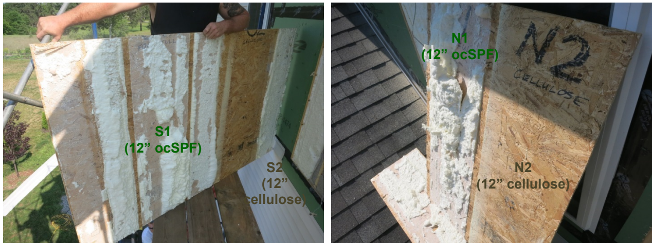
Figure 15: Sheathing conditions at south-facing (left) and north-facing (right) walls
