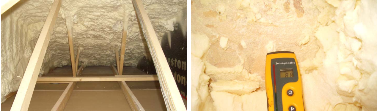
Figure 22: Unvented cathedralized attic in Coquitlam test facility (left) and sheathing MC measurement (right)
