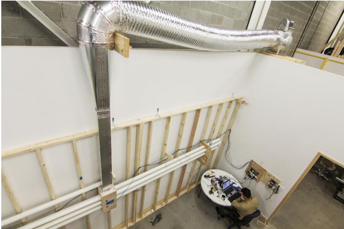
Figure 5. Testing a side outlet manifold configuration
