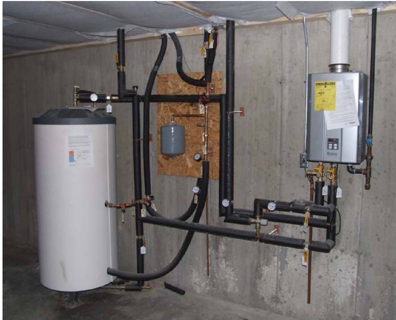
Figure 5. Solar tank and auxiliary water heater in a WWSV basement
