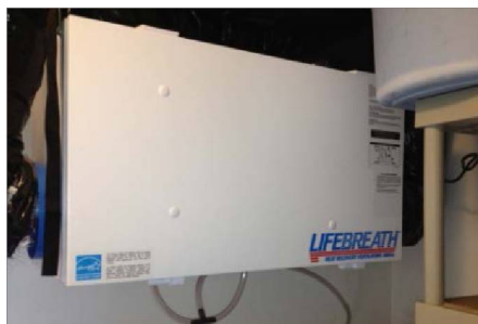
Limited access to changing filters (homeowner issues)
