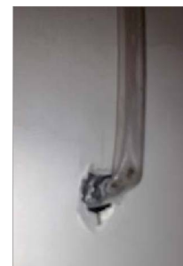
Kink in condensate drain (installer issues)
