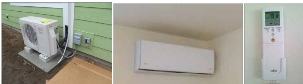
Figure 4. Outdoor and indoor DHP units and remote thermostat in living room
