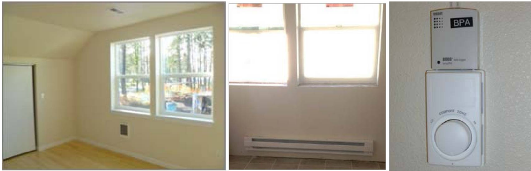
Figure 5. ER, fan, and baseboard types and hard-wired thermostat in living room with temperature/RH data logger
