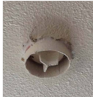
Installed sprinkler housing at dry wall stage prior to indoor head installed
