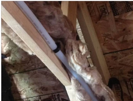
Sprinkler plumbing with tented insulation required by fire marshal
