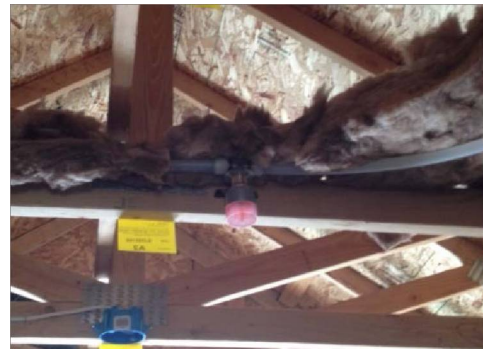
Sprinkler insulation freeze-protection tent over pipe
