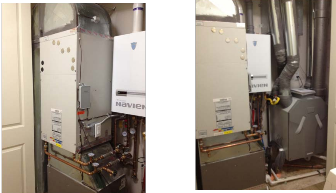
Figure 17. Mechanical closet with the air handling unit and water heater (left) and the ERV (right)
