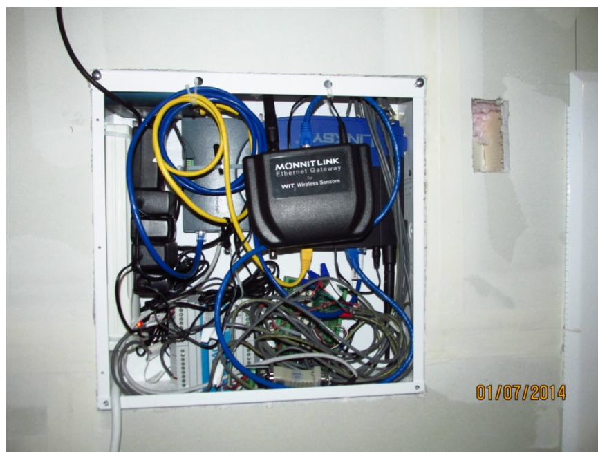
Figure 25. Data logging control center in the basement of the Passive House
