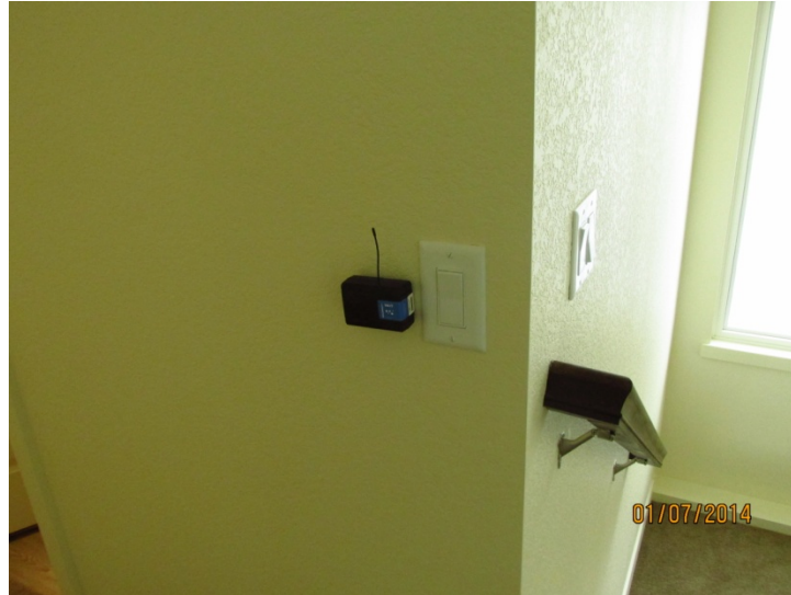
Figure 26. Wireless temperature and relative humidity sensor location on the second floor of the Passive House
