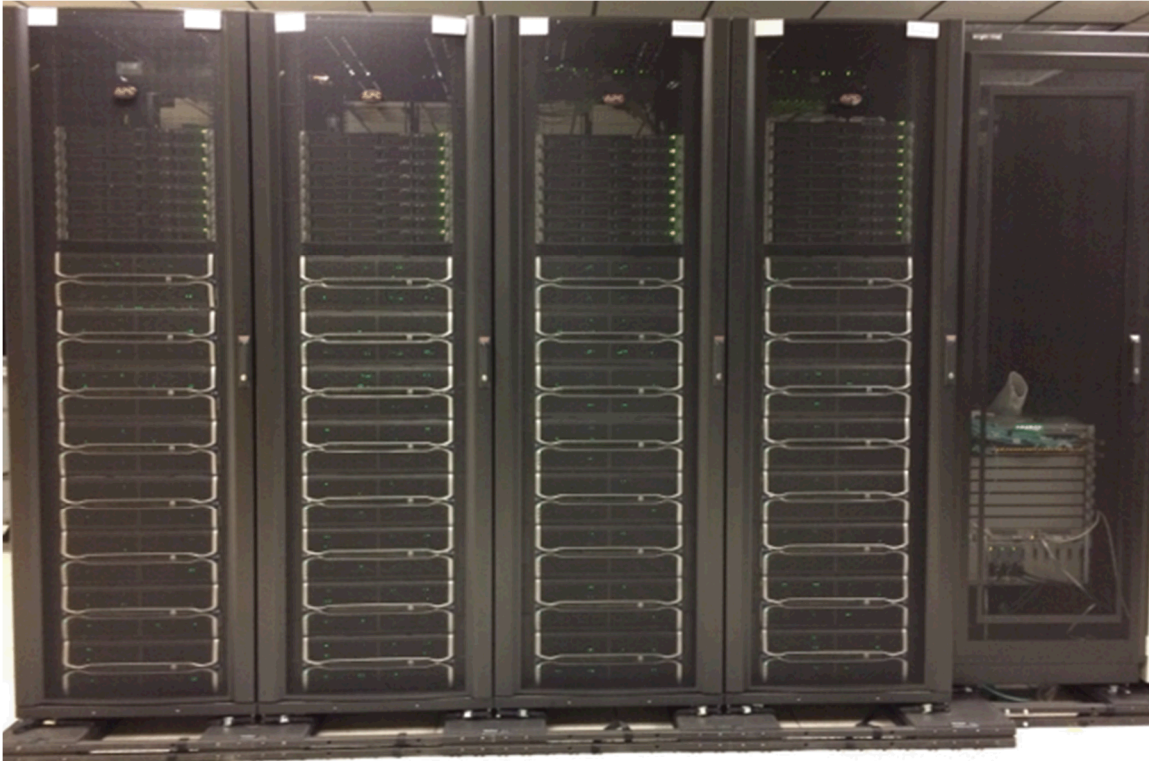
Figure 1: Yuban Archive Disk Rack Storage Scalable Units (four RSSUs) plus 40GbE switch on the right (not pictured: Osprey 6 RSSUs plus switch rack)
