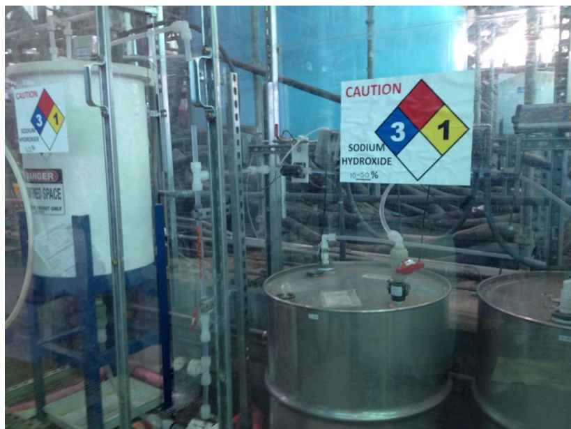
Figure 2-15 Caustic feed tank and product drums
