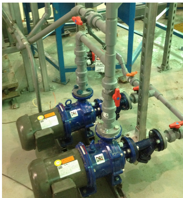
Figure 2-14 Centrifugal pumps installed in parallel for all electrolytes
