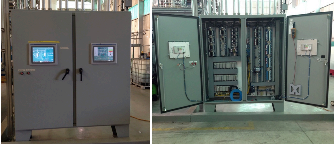
Figure 2-20 Programmable Logic Controller (PLC) and instrumentation cabinet for the ABLE subsystem
