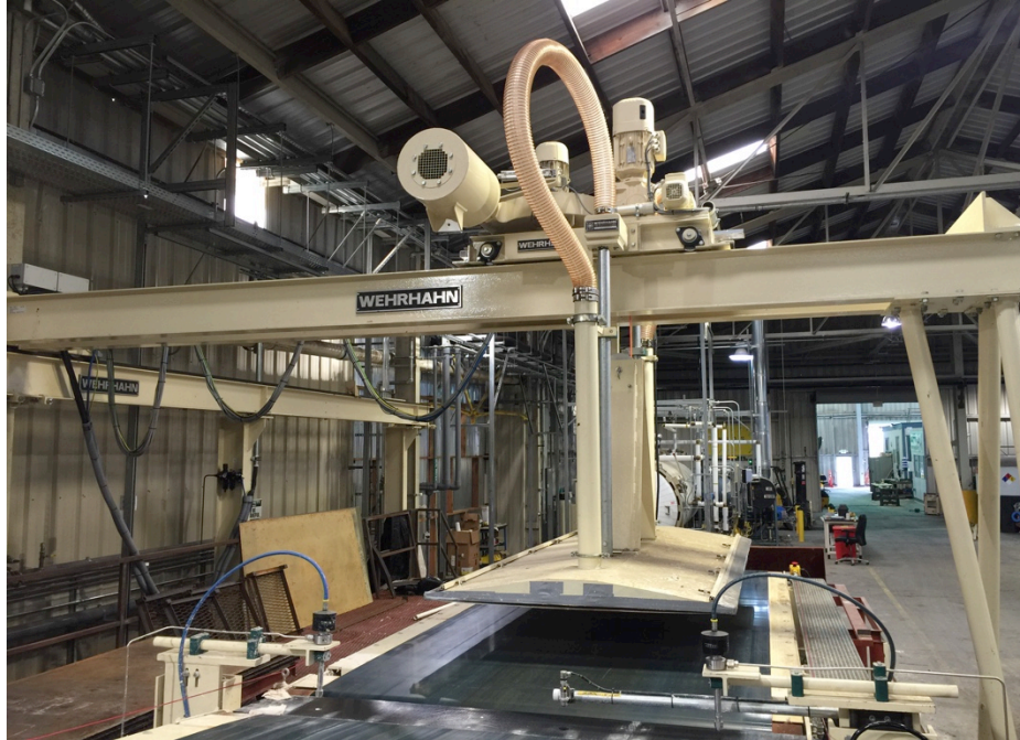
Figure 2-33 Green board stacking device on the Calera fiber cement board production plant
