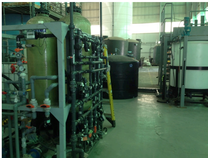
Figure 2-13 Brine preparation tanks and ion exchange unit
