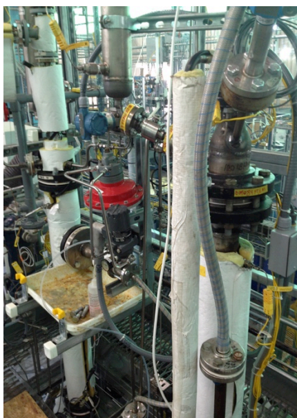
Figure 2-17 Picture of top of catalysis reactor
