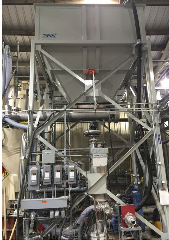
Figure 2-27 Carbonate silo used in the Fiber Cement Board Production Subsystem
