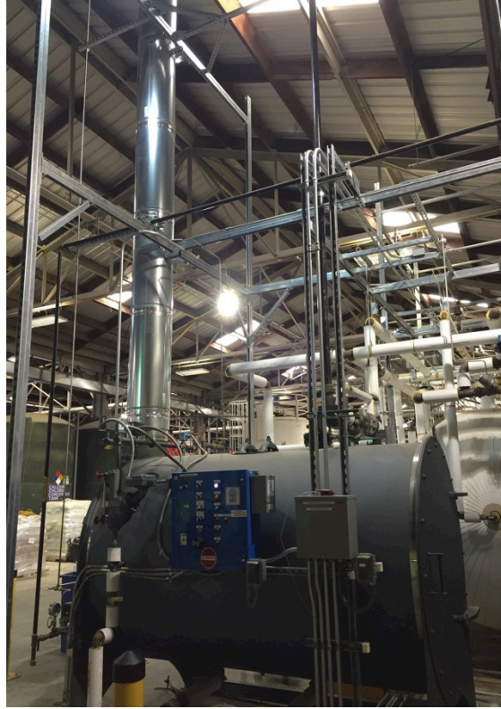
Figure 2-36 Steam boiler system supplied steam for autoclave unit fired with propane
