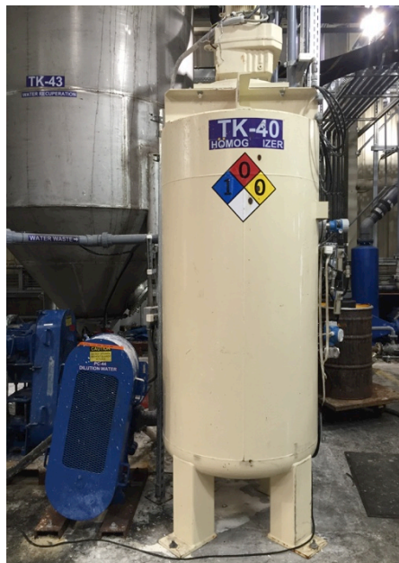
Figure 2-29 Homogenizer Tank used for final adjustments of water content, required flocculants, mixed fresh slurry, recycled rejects and cut-off material in preparation for target slurry density for the sheet production
