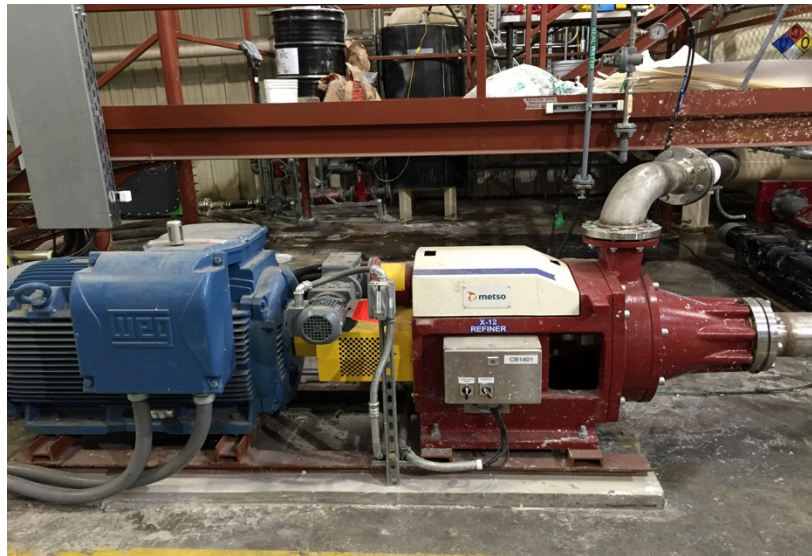
Figure 2-25 Cellulose Refiner used in the Fiber Cement Board Production Subsystem
