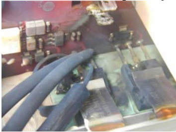
Figure 8. Residential inverter failure occurred while restarting after ~8hrs of non-unity operation.
