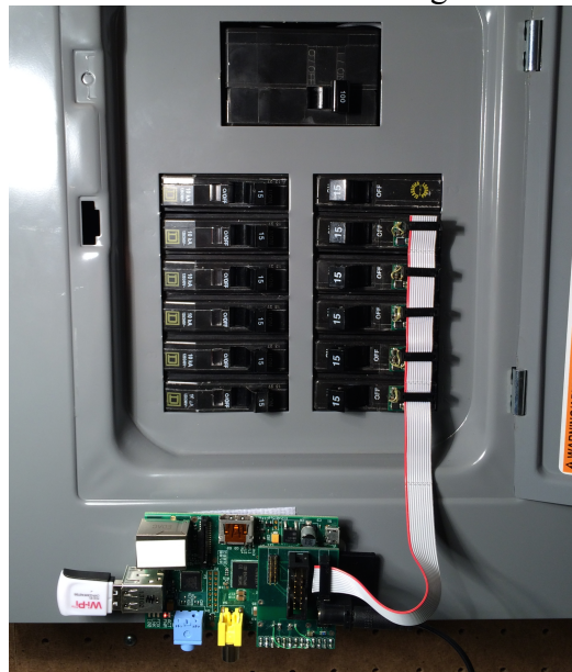
Figure 10 Photo of installation of SEM on a residential circuit breaker panel. The wireless interface board is mounted at the bottom of the panel and SEMs are mounted to five breakers.
