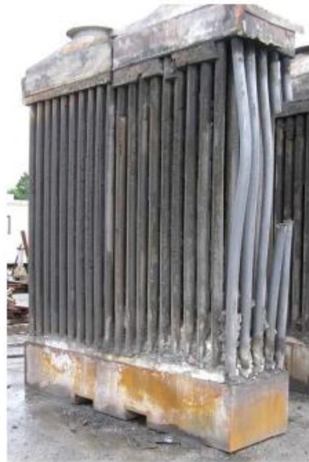
Figure 2-1. Recuperator used on an aluminum melting furnace. Note bent and broken tubes in the first row and missing refractory on the upper end of the tubes [4].
