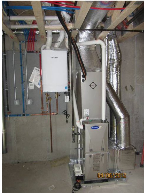
Figure 12. Air handler in basement
