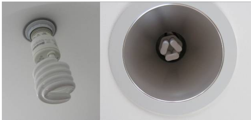
Figure 10. CFL and pin-based lighting installed
