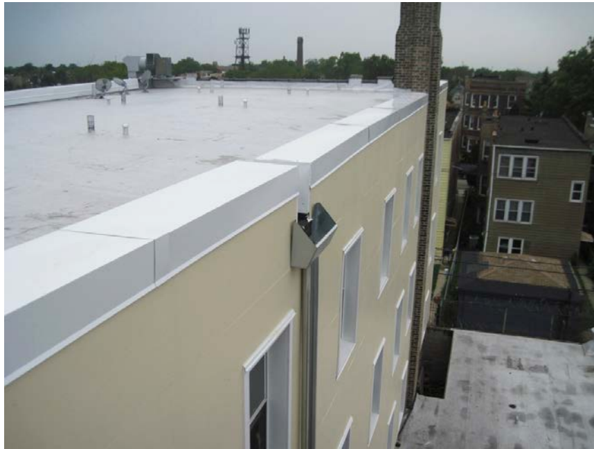
Figure 53. Visible butt joints in the finished wall
