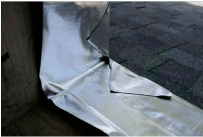
2011-08-28 – Gap in corner flashing
