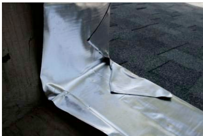
2011-08-28 – Gap in corner flashing
