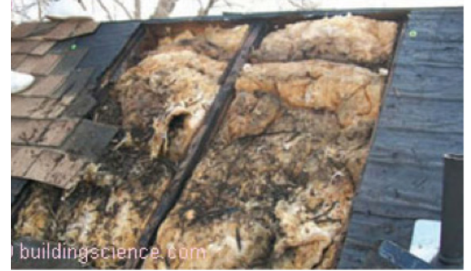
Moldy fiberglass batts. The fiberglass insulation in this unvented cathedral ceiling absorbed moisture, leading to mold and wood damage. Building America scientists do not recommend using fiberglass or cellulose in a cathedral ceiling or flat roof, unless rigid or spray foam insulation is installed above the fiber to form an air and moisture barrier (Photo source: BSC).
