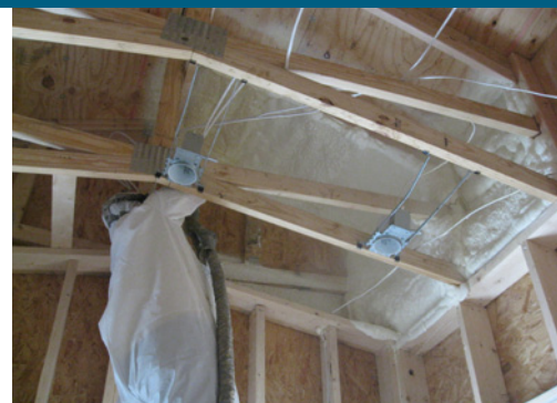
Polyurethane foam insulation. Leave the installation of spray foam to trained professionals. Toxic gases emitted during application are hazardous to skin, eyes, and lungs (Photo Source: NAHB).
