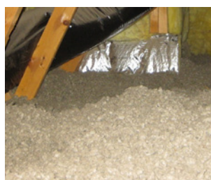
Loose fiberglass insulation
