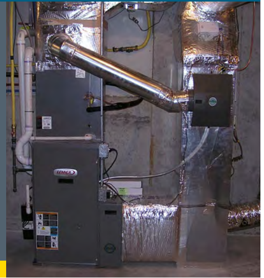
High-efficiency, sealed-combustion HVAC equipment increases savings and works well with the tighter building envelope of Building America homes. (Photo Source: BSC)
