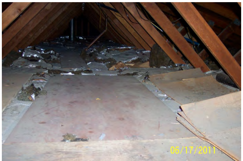
Attic is only insulated to R-11.
