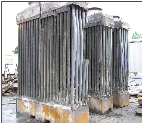
Figure 3 - Abandoned Recuperator from an - Aluminum Melting Furnace (Source: ORNL)
