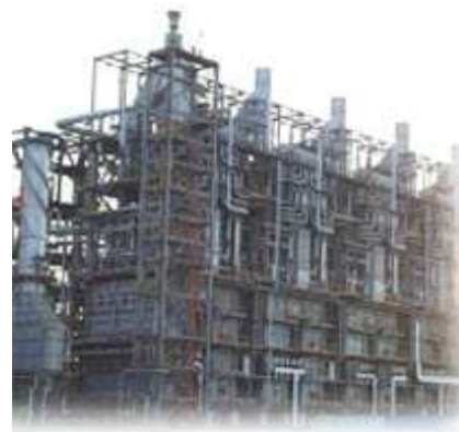
Figure 28 - Ethylene Furnace (Source: Sela Fluid)
