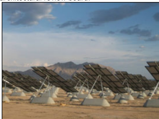
Figure 3. Nellis AFB PV Installation
