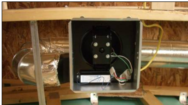
Figure 44. Improperly installed ventilation fan
