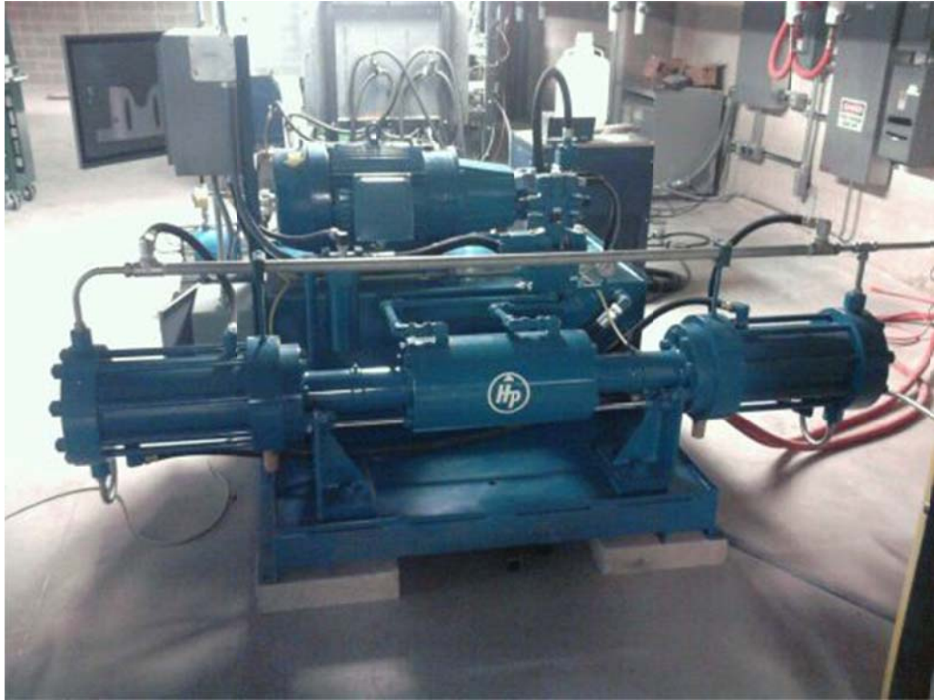
Figure 9. Single Stage HydroPac compressor used in UW-Madison facility.
