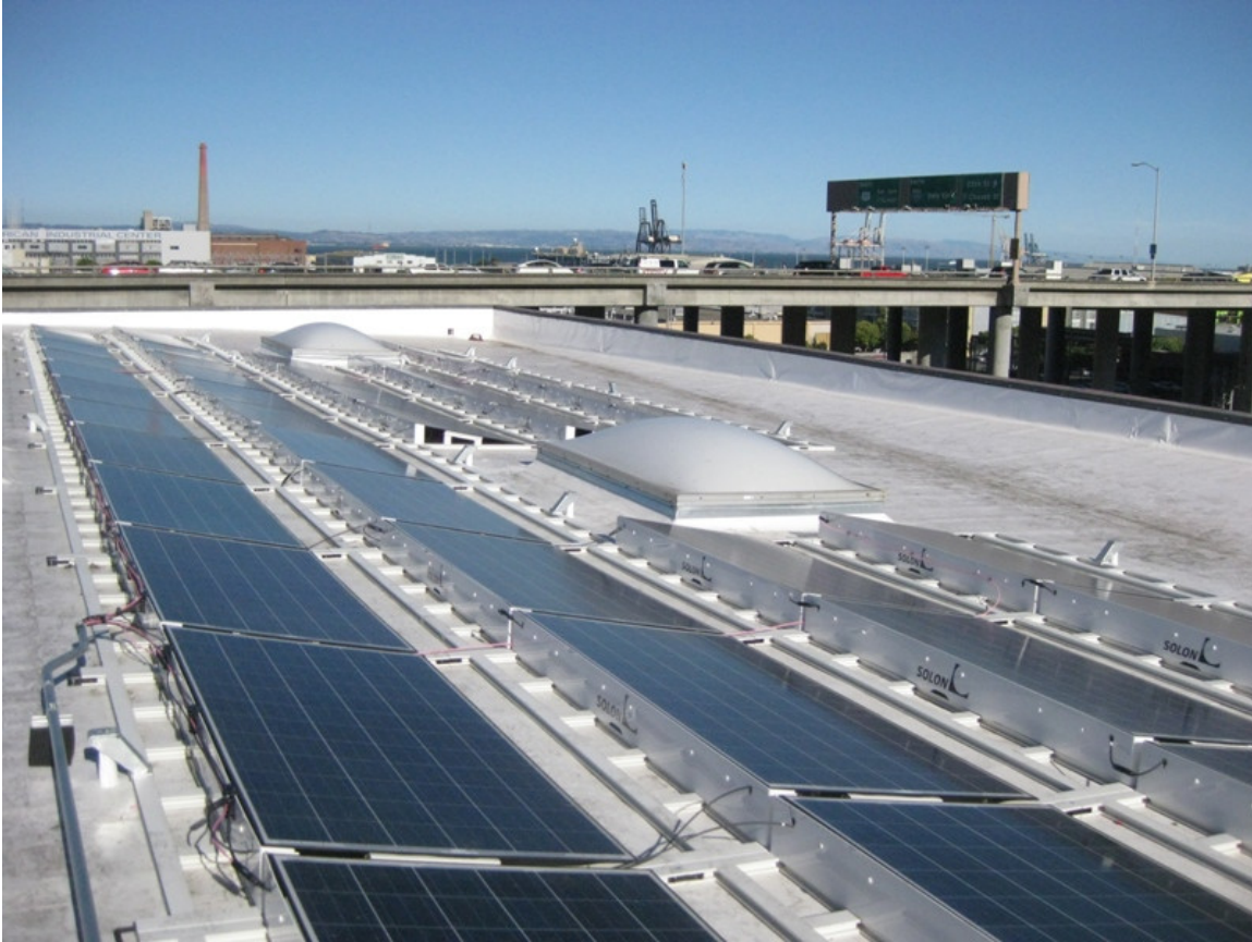
Solon SOLquick PV system installed at MUNI Ways & Structures facility, San Francisco
