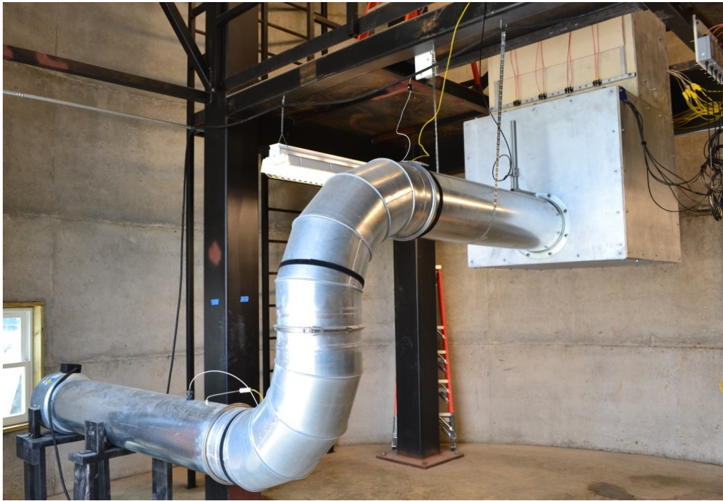
Figure 9 - Inlet plenum and piping.
