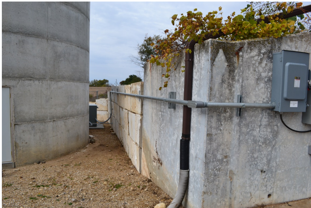
Figure 122 – Electrical line from Stoughton facility to silo.
