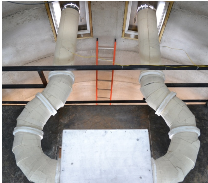
Figure 22 – Insulation on the two exhaust ducts.
