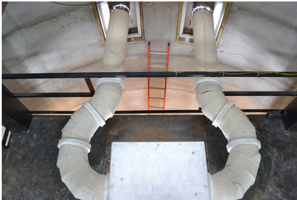
Figure 116 – Exhaust ducts insulation.
