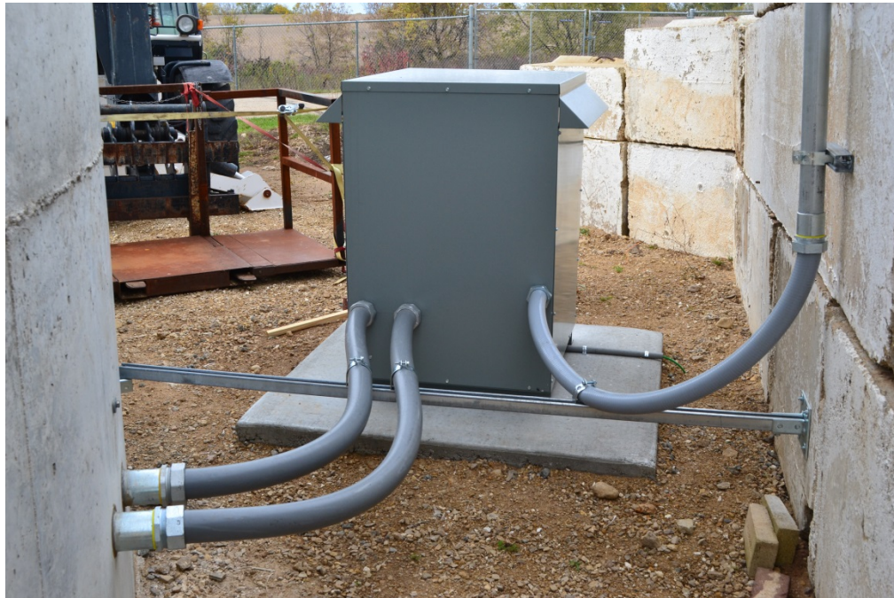
Figure 121 – Transformer outside silo.
