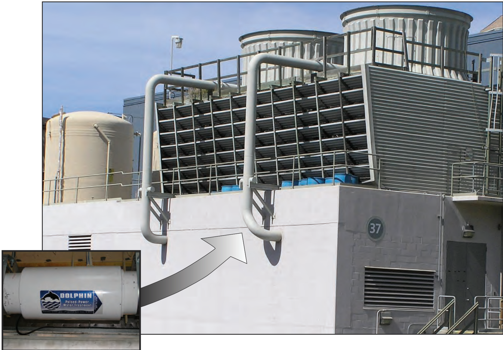
A nonchemical (Dolphin) water treatment system was installed at the Building 37 cooling tower, which eliminated use of chemicals to control biological fouling, scale, and corrosion
