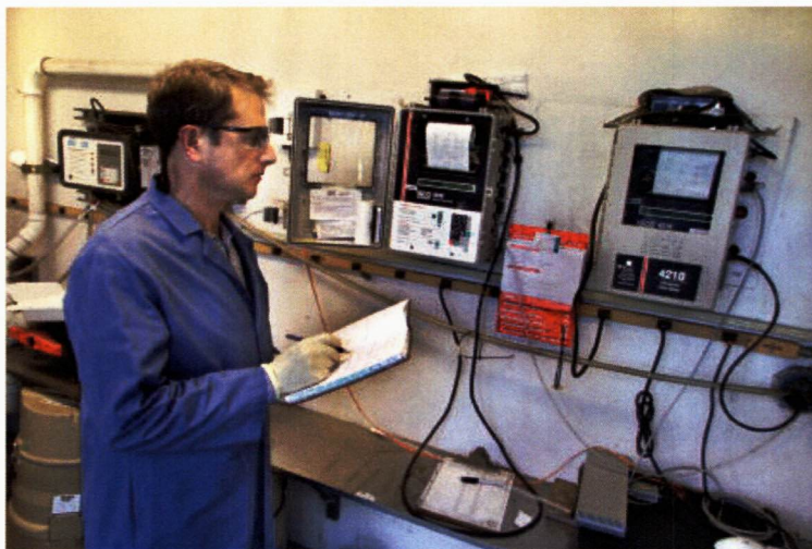
Automatic water-sampling and flow-measurement instruments at the Hearst Sewer Monitoring Station
