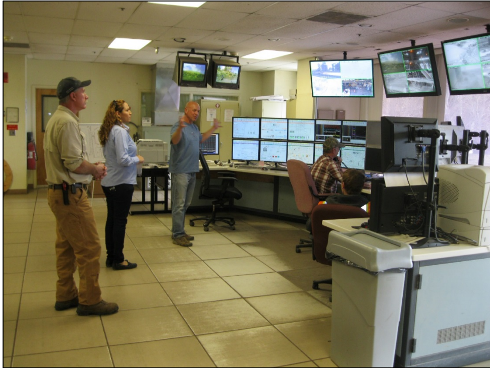
Two operators run the plant using computerized process controls.
