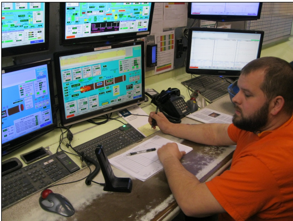
Nevada Cement Control Room
