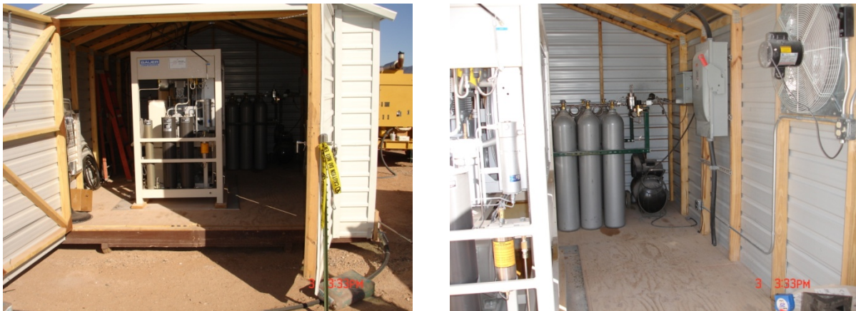
Figures H-6a and H-6b. Air compressor building.
