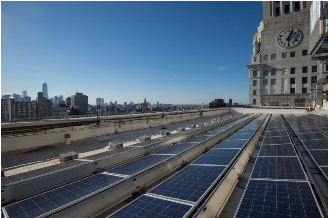
Figure 4-9. PV Installation on Con Edison's Headquarters
