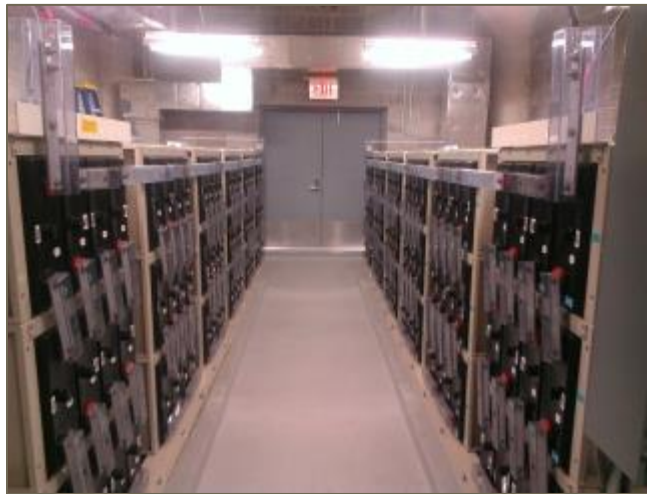
Figure A-64. 720 kWh Battery Installation at BAT
