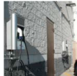
EV Charging Level 2 and Level 3
