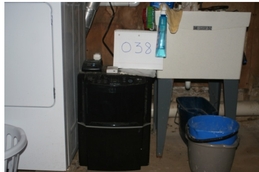
Figure 11-5 Dehumidifier with clothes dryer
