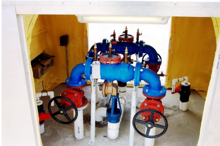
Hot Box Valves SNL Area 3 to USAF Area 10 PWS Connections
