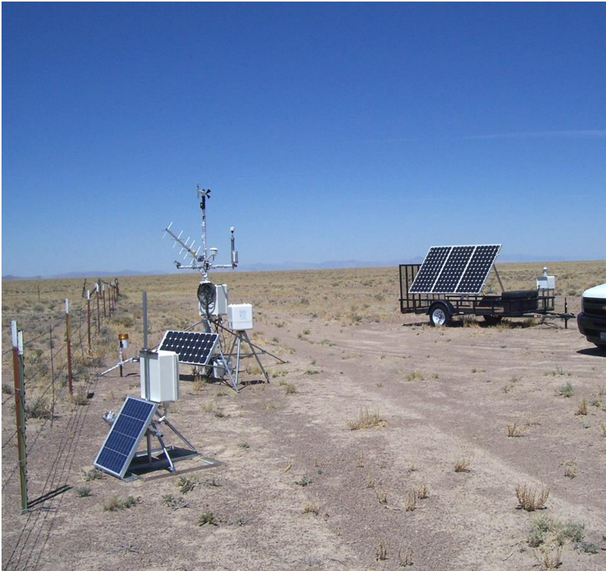
FIGURE 1-5. The solar powered air sampler, saltation sensor, and meteorological tower (center right, foreground left, center left, respectively) at Station 402 are located along the north fence that bounds the Clean Slate 1 contamination area.
