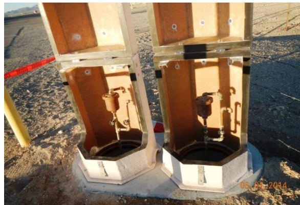
Heated Enclosures for raised Air Vacuum Valves
