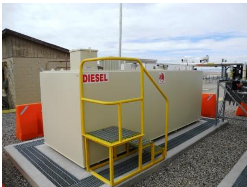
2,000 Gallon Diesel Fuel Tank for TTR Area 3 Emergency Backup Generator
