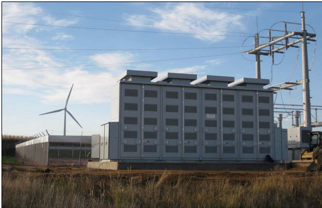
Figure 34. Xcel Battery Supplementing Wind Turbines, Lucerne, MN
