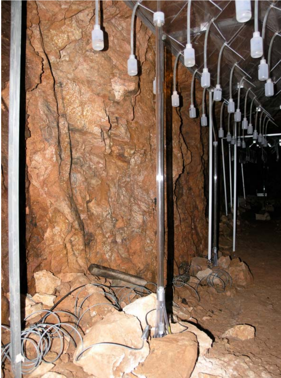
Fig. 3 Array of collection bins and instrumented collection columns (sites 24C, 18A, 8C, and 3C, from foreground to background) within adit seepage collection system
