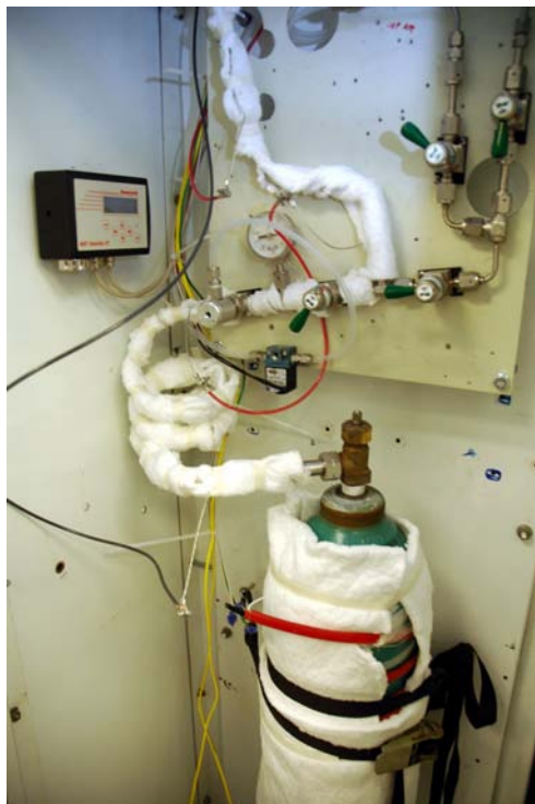
Figure 3.16: The hydrogen fluoride cylinder in the toxic gas cabinet showing the heated, vent, and purge lines. All hydrogen fluoride containing lines were oriented atleast partially vertically so that liquid hydrogen fluoride could drain.
