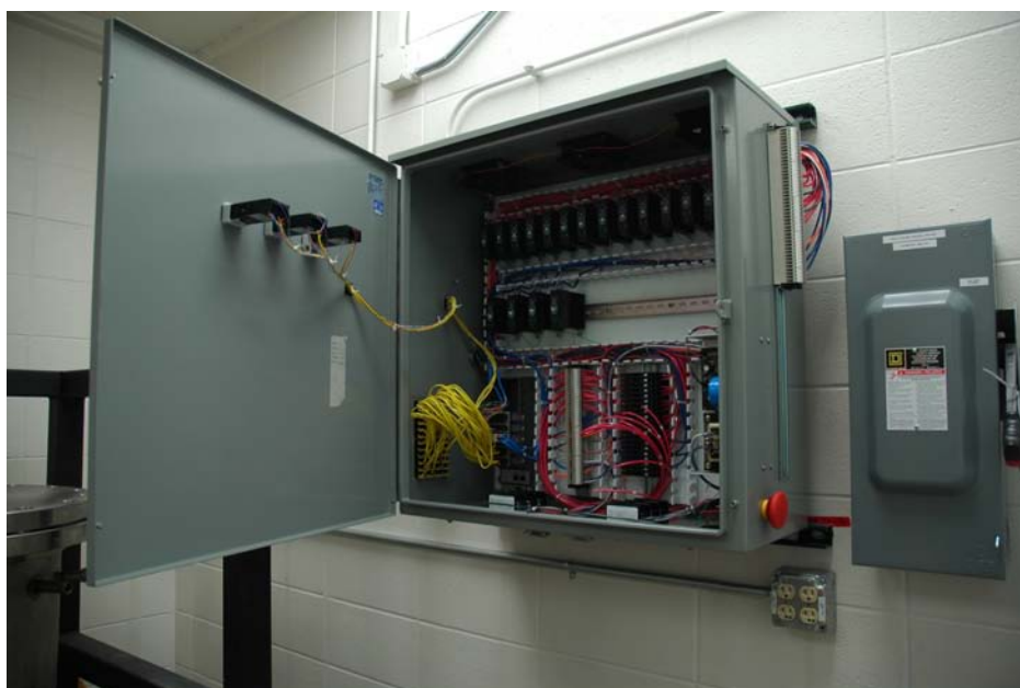
Figure 3.14: The first version of the electrical box. Four more AC SSRs were added after this picture was taken.
