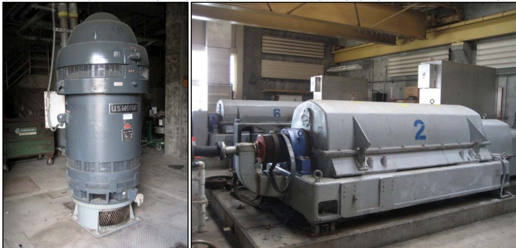
Figure 4: Examples of lift pumps (left) and centrifuges (right) at the Southeast plant
