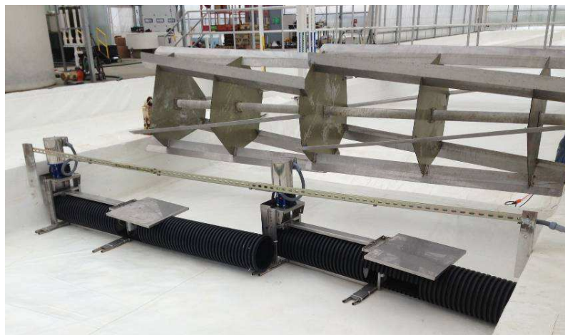
Figure 43. Screw pumps installed in Pond 3
