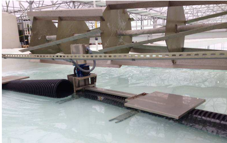
Figure 44. Intake pipe floating to surface
