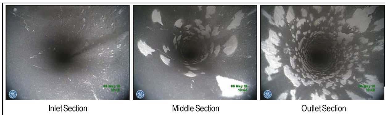
Figure 46. Post-Run Inspection of Primary Gas Cooler Tubes.
