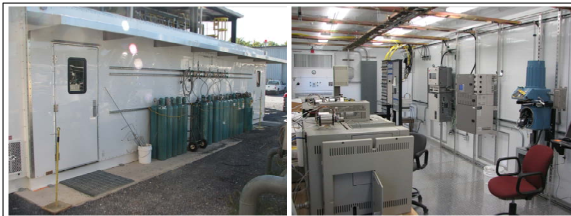
Figure 5. Gas Analyzer Building for the Syngas Conditioning Unit.
