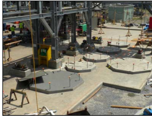
Figure 36. BOP Area Foundation with Chemical Storage Tank and Pump Pads.
