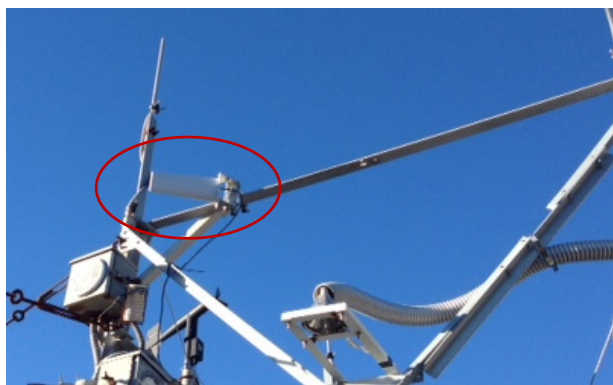
Figure 9: New redundant 3G cellular network Internet link pointing toward Horta. The antenna (red circle) is installed at the northern corner of the station top structure.
