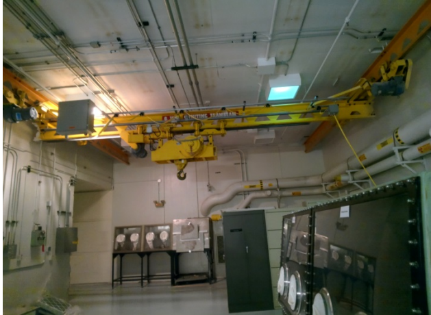
Figure 12 Glove boxes, overhead piping, and gantry crane
