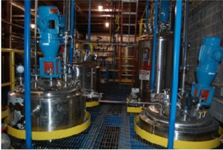
Figure 3-13: Top of skid view of fermentation process. Fermentor C (left) and Beerwell tank (right) in the foreground. Fermentor B (left) and Fermentor A (right) in the background.
