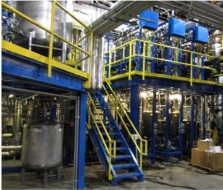
Figure 3-15: MSE skid installed at ADM EWA.
