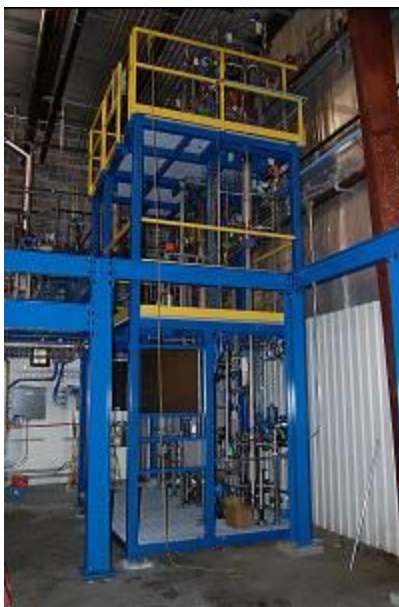
Figure 3-17: Distillation skid installation at EWA (2012).
