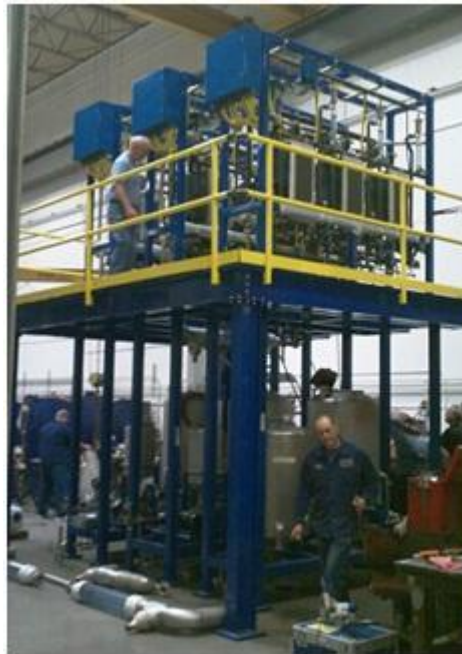
Figure 3-14: MSE skid assembly at Anderson-Dahlen.
