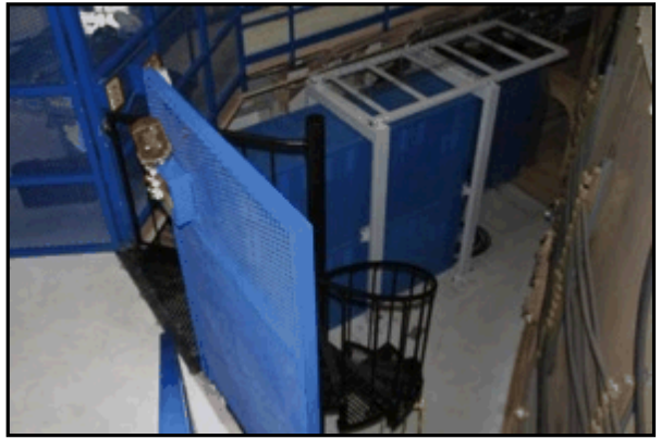
Capacitor bank system on Z 900 kJ, 8 mF, 15 kV
