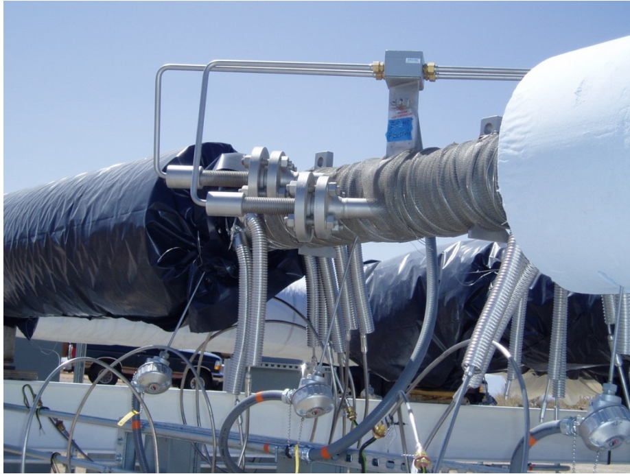
Figure 1. A flowmeter in MSTL, shown during construction, remains uninsulated and is contrasted with the highly-insulated piping.
